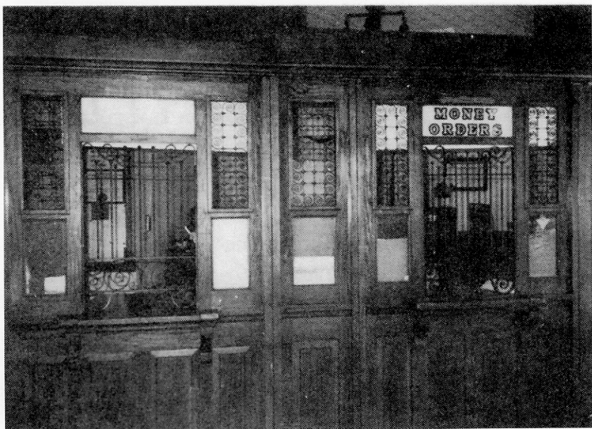
Interior service windows, still guarded with cast-iron decorative bars and surrounded with varnished wood paneling
