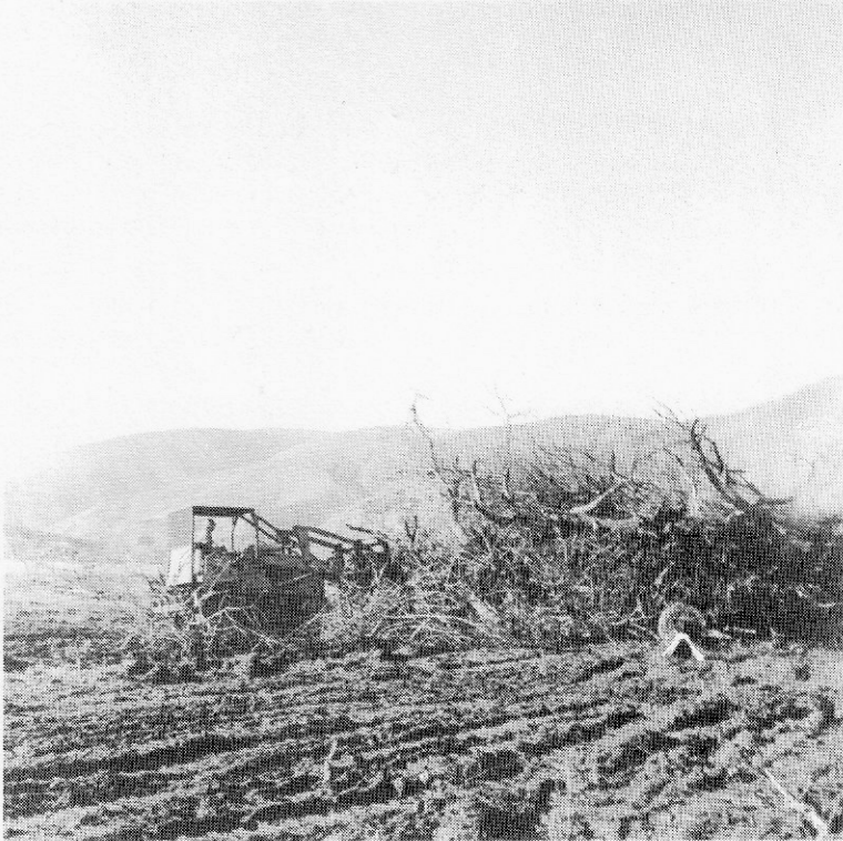
Herb Snelgrove pushes trees into piles for burning in 1967 as clearing of Snake river orchards began in the Lower Granite dam reservoir. This ended the once thriving industry in Whitman county.
